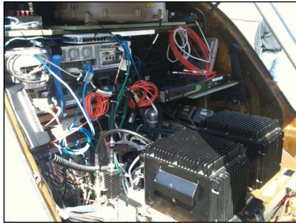
Figure 1: Interior of Proxy's payload bay showing a payload of 5 sensors and processors, 5 communications systems, and Proxy's Virtual Pilot.
